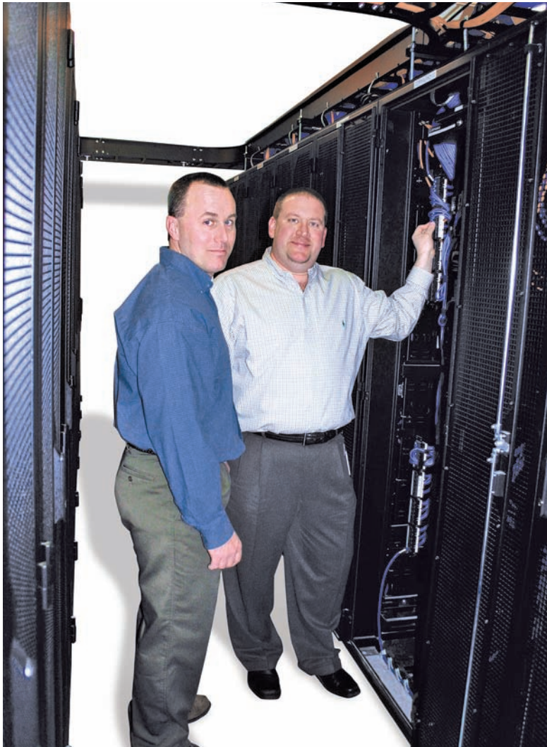
Randall Rossetti, president of Innovative Cabling Systems, and Michael French, network services manager, corporate information systems, for PerkinElmer, check the cabling connections in the corporate data center.
